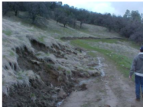
Slumping Along Road
